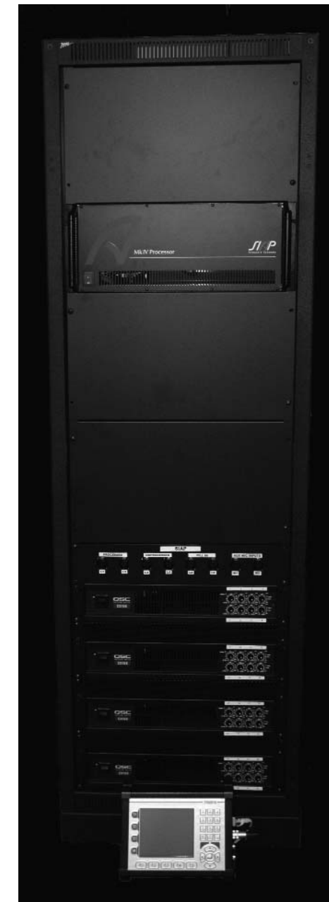
Figure 3. Rack mounted 32 output SIAP Processor, processed, unprocessed, fill and aux inputs below that, four 8-channel amplifiers, plus keypad selection panel below that
